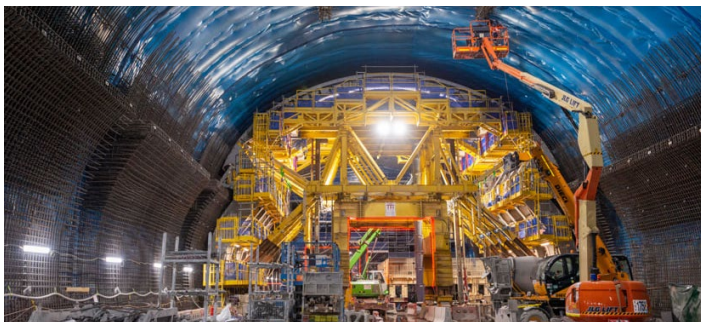
The Roma Street cavern shows the complexity of the two-tunnel subway line.
